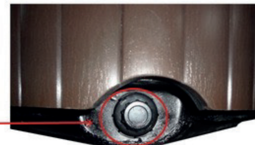
corner drain valve
