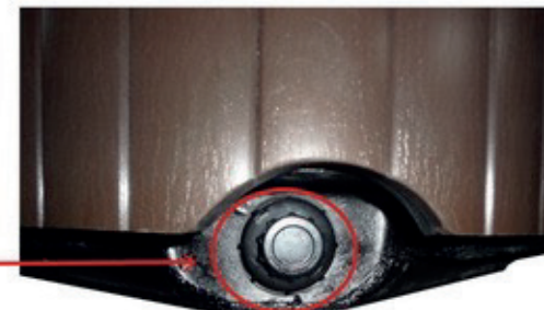
corner drain valve
